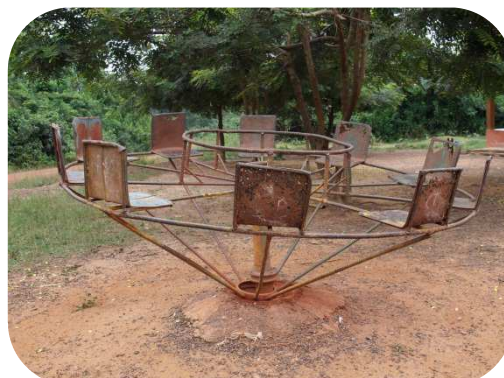
Playground with rusty equipment, Wuruye
